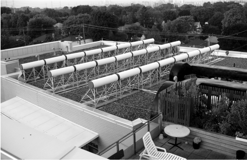
FIGURE 12.4 Solar Thermal Evacuated Tube Technology installed on the rooftop of Wilmar Court
